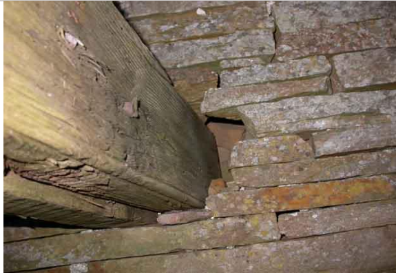
Internal gaps near loft beam
