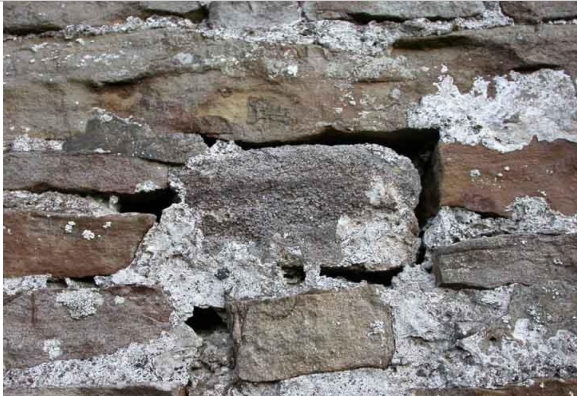
Missing stone mortar
