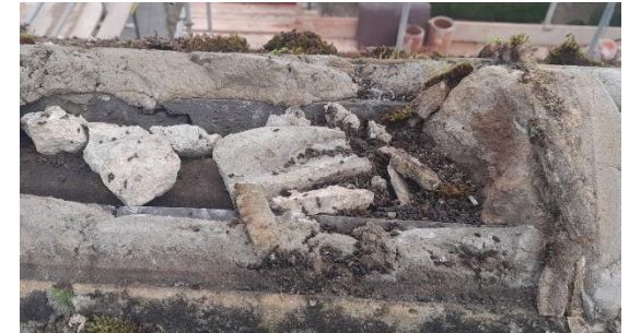
Bat droppings under ridge tile
